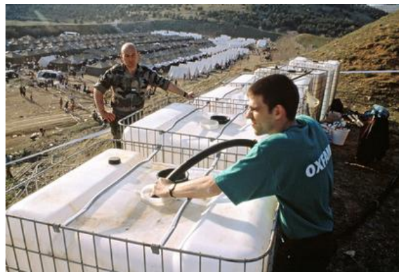
OXFAM worker installs a water supply system at Stankovac; Photo taken by HJ Davies. http://downloads.unmultimedia.org/photo/medium/763/76370.jpg
